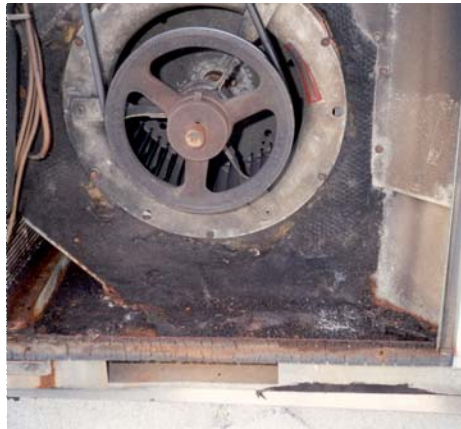
Internal damage caused by P-traps includes systems that are wet, dirty, and filled with fungi causing poor air quality.
